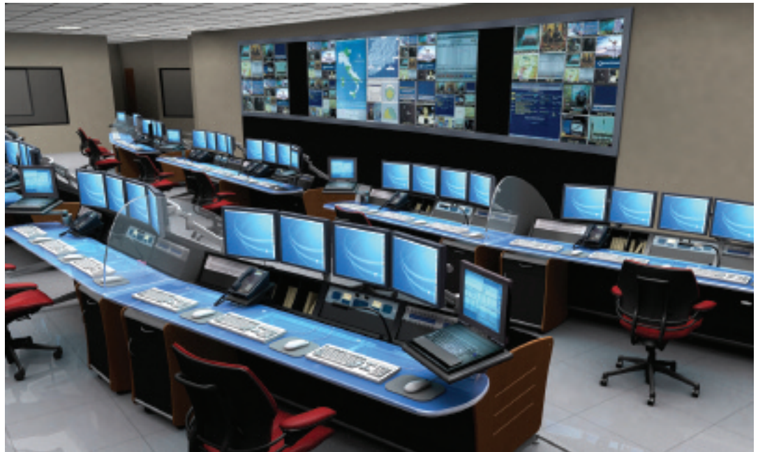
Some of Diversified Systems' projects resemble IT jobs more than AV integration projects. For instance, the company specified a network operation center for Qualcomm in San Diego, a site that harvests local news video from all over and encodes it for delivery to mobile devices.
